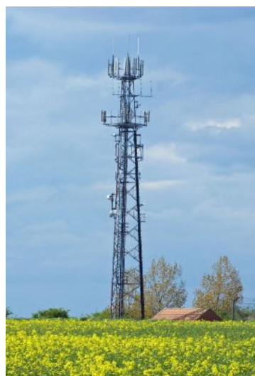
Example of cellular macro site
